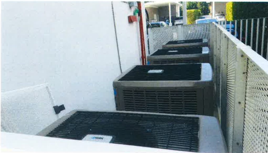
VILLA 1 – A/C ON NORTH SIDE 2-20-2019
