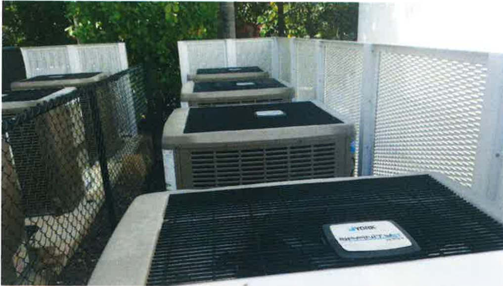
VILLA 6 – A/C ON SOUTH SIDE 2-20-2019
