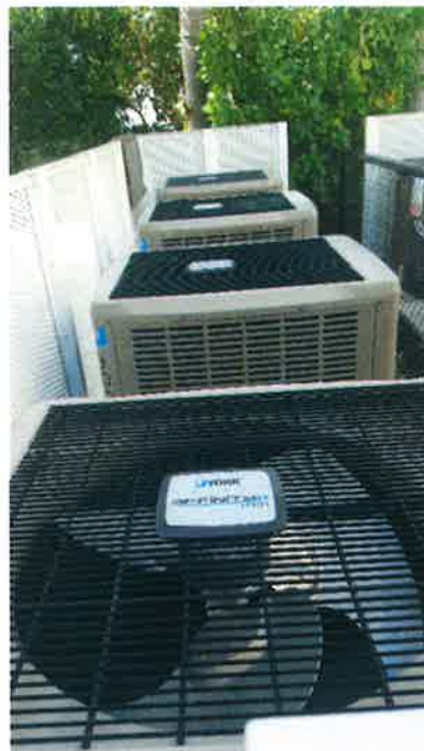
VILLA 7 – A/C ON NORTH SIDE 2-20-2019
