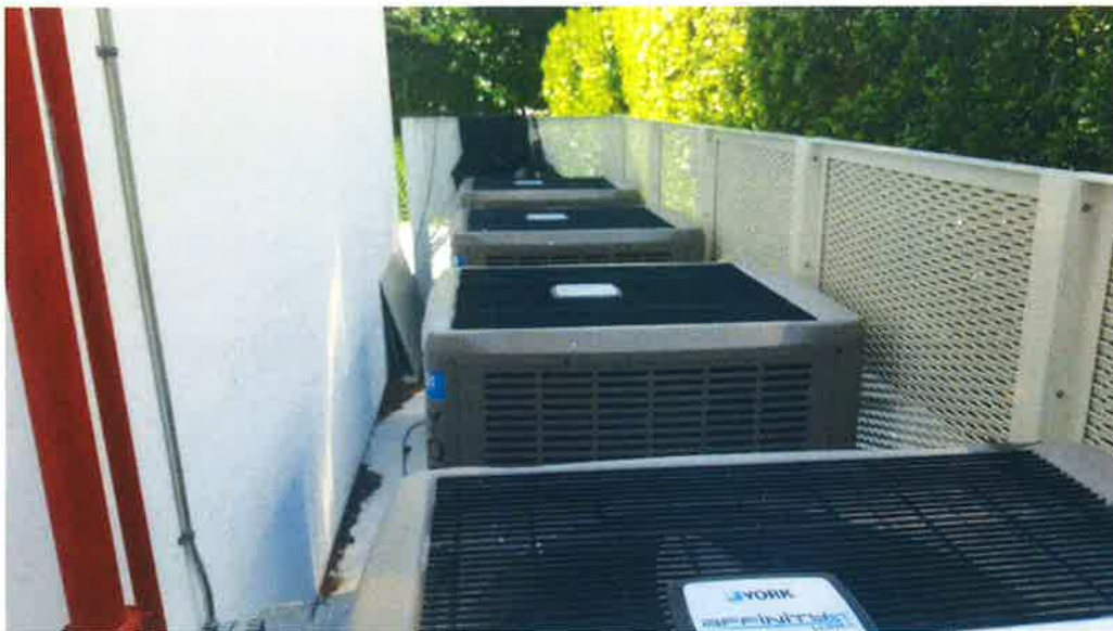
VILLA 9 – A/C ON NORTH SIDE 2-20-2019
