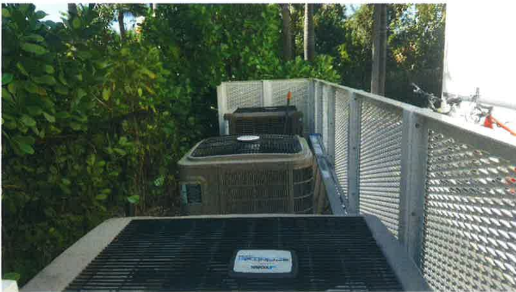
VILLA 10 – A/C ON SOUTH SIDE 2-20-2019
