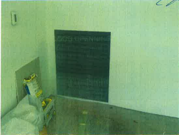
FLOOD OPENNING VIEW
